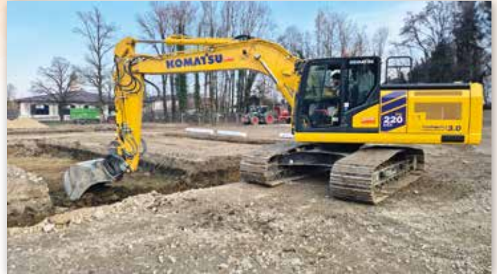
Precision work with the Komatsu PC220LCi-12: It is the first excavator in its class to be fitted with IMC 3.0 as standard.
